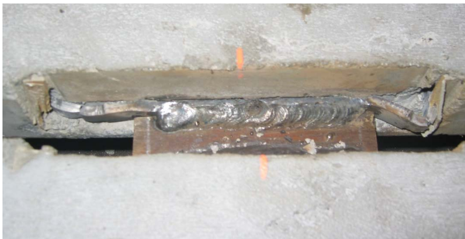
Figure 14: Damage at end of test
