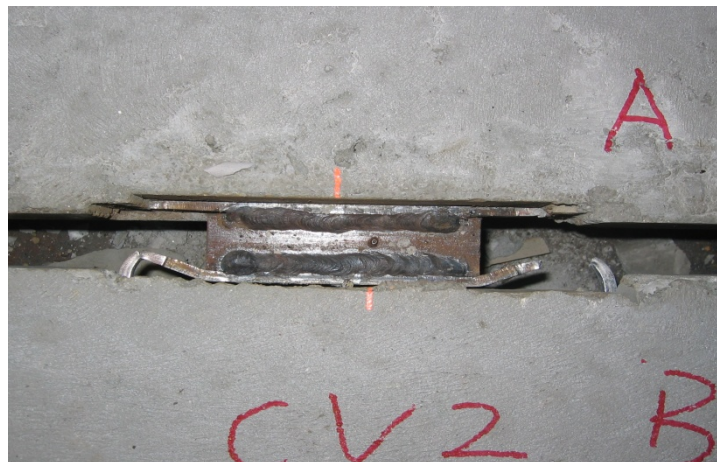
Figure 18: Damage at end of test
