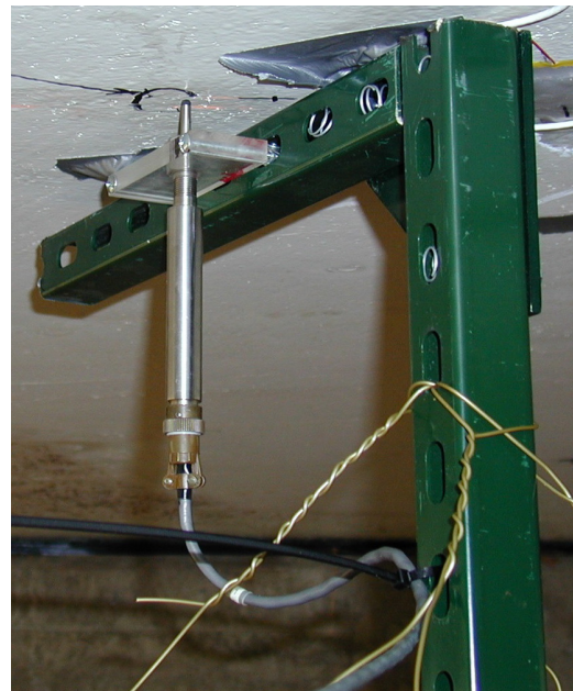
Figure 4: Typical Displacement Sensor Installation
