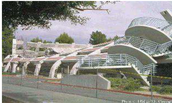
Collapsed Northridge Parking Structure. Photo Courtesy of U.S. Geological Survey.
