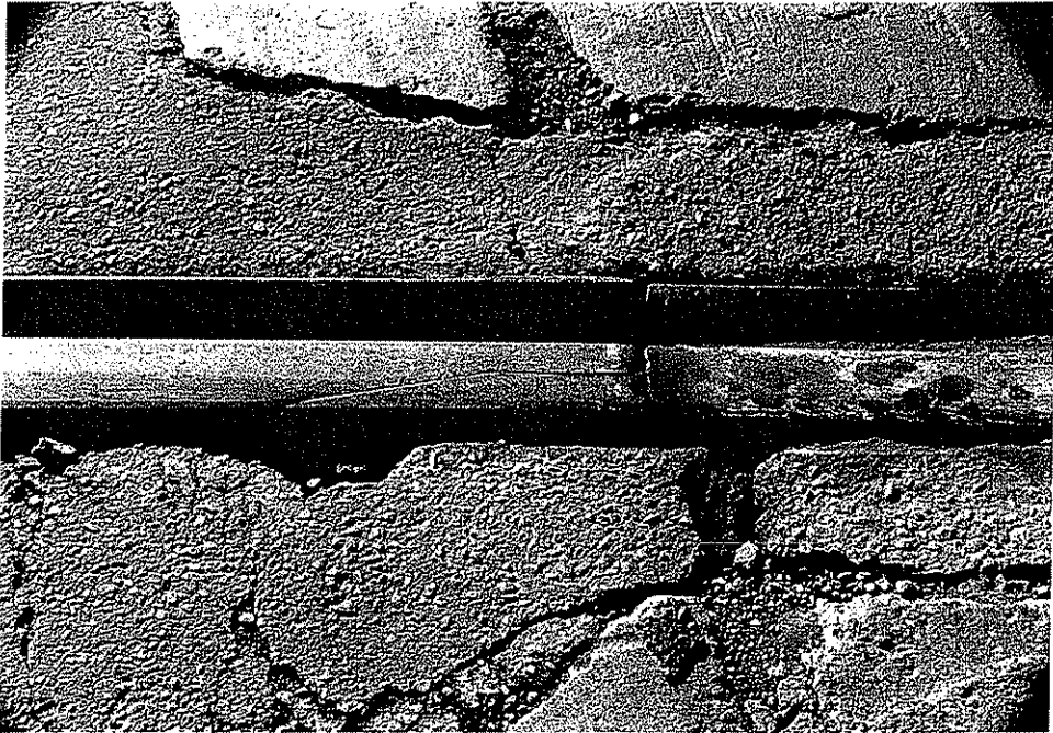
Figure 16: Mitered Rail Joint on Inbound Track in Span 10 (2/99/15-9)
