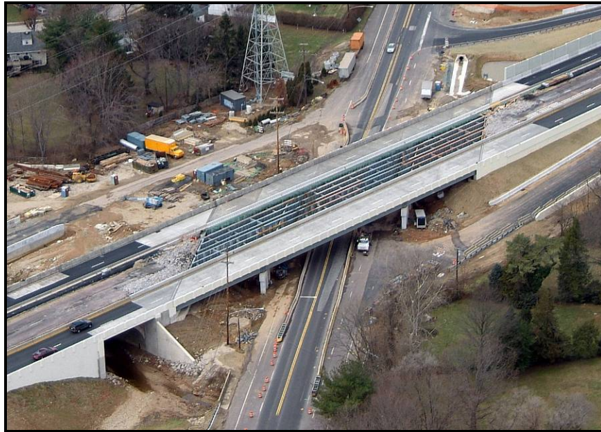
Figure 1.1 – Aerial view of SR309 over Church Road Bridge during widening construction looking northwest (Stage 5 under construction) [PennDOT 2007]
