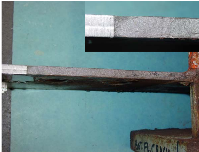
Figure 12 - Crack Arrest Region in the Lateral Gusset Plate.
