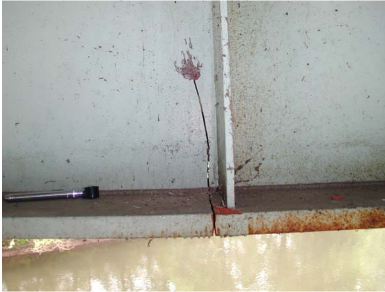
Figure 1 - Fractured Bottom Flange of Girder and Arrested Web Fracture. (Photo Courtesy of Gannett Fleming)
