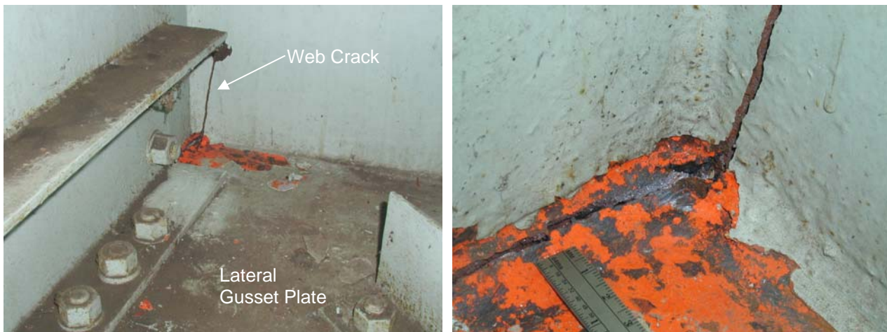
Figure 2 - View of Lateral Gusset Plate Connection and Fracture at the Weld Intersection of the Gusset and Vertical Stiffener Plates to the Web. (Photos courtesy of Gannett Fleming)
