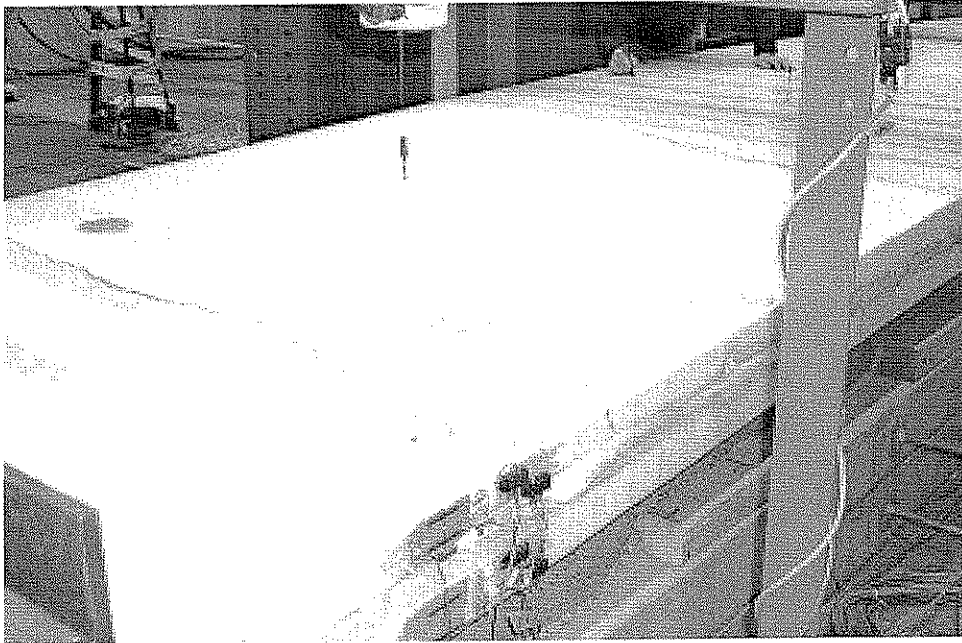
Figure 4.32 Cracks 2, 6, and 7, which formed around a 1 ft. square solid concrete region.
