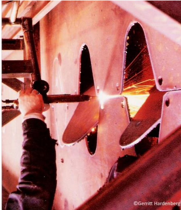
Figure 27 Burning of rib profiles in floor beam web (reproduced from Gerritt Hardenberg)
