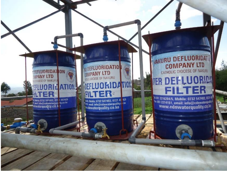
Figure 11.7. HAP filters installed by JB Drilling in a treatment system outside Nakuru.
