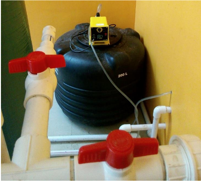
Figure 3.13. Close-up of 200 L chemical dosing tank behind Column I with chemical-resistant pump at the Baduria treatment system.
