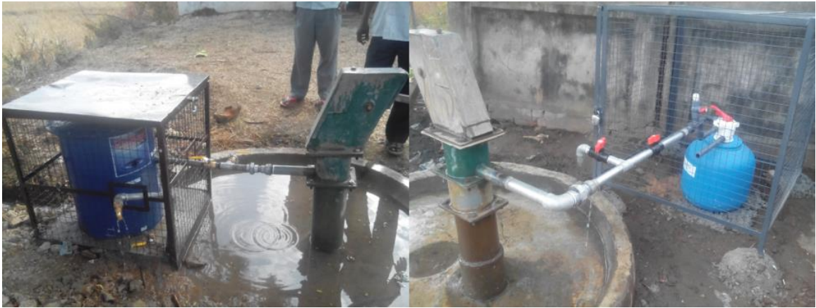
Figure 7.5. Fluoride removal systems from HES (L, OxiMax) and Ion Exchange (R, Indion-RS-F). Note the much smaller volume of HES and Indion systems.
