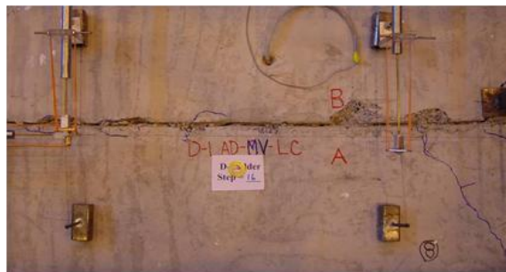
Figure 4.24. Damage state at 0.33-in shear opening
