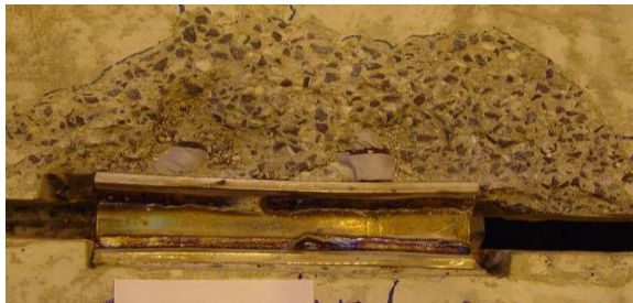
Figure 4.38. Damage state at 0.75-in shear opening
