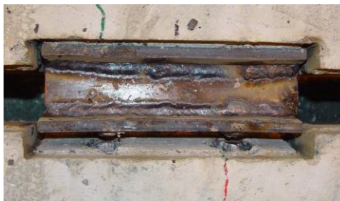
Figure 4.16. Damage state at 0.39-in tensile opening
