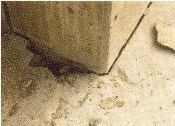
(a). cracking and fracture of connections between wall and double-tees
