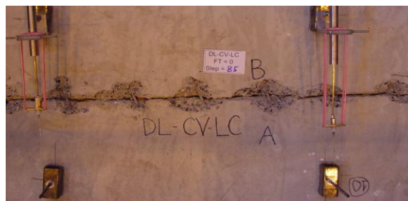
Figure 4.26. Damage state at 0.77-in shear opening
