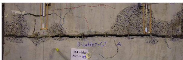
Figure 4.11. Damage state at 3.0-in tensile opening
