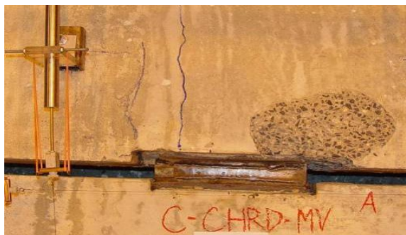
Figure 4.32. Damage state at 0.75-in shear opening
