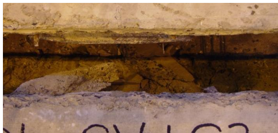
Figure 4.30. Damage state at 1.08-in shear opening
