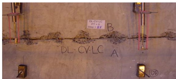
Figure 4.29. Damage state at 1.0-in shear opening
