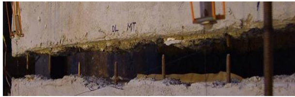
Figure 4.10. Damage state at 2.5-in tensile opening
