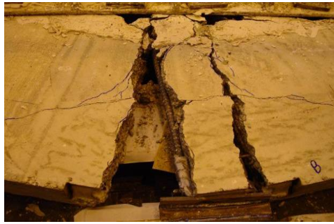
Figure 4.15. Damage state at 5.0-in tensile opening
