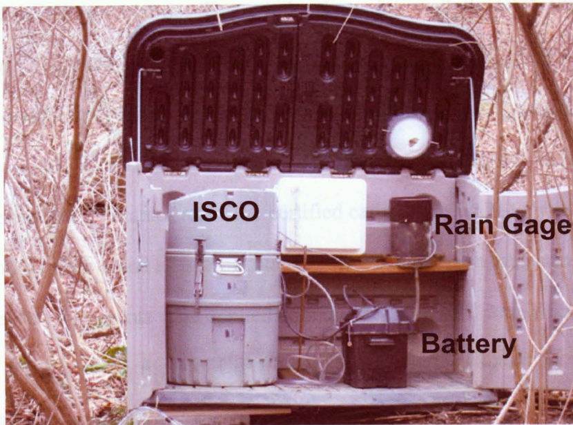
Figure 11: A photograph of one of the garden-shed enclosures containing an ISCO automated sampler, the rain gage for triggering storm sampling, and a battery to power the system.
