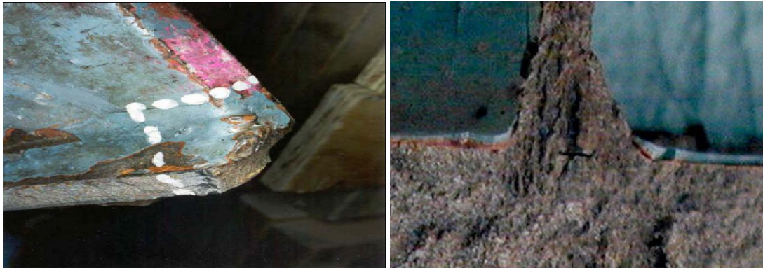
Figure 1.3 Fracture in highly constrained welded plate girders. [8]
