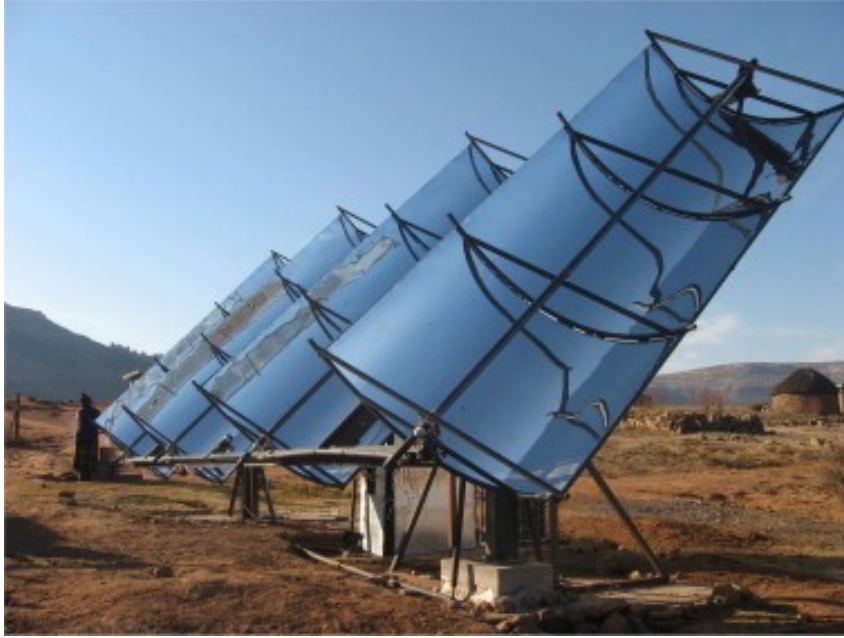
Figure 2.3. Solar ORC prototype installed by STG in Lesotho [10]
