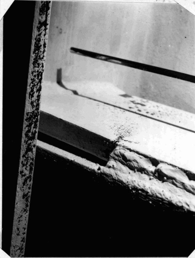
Fig. 20(a) - Top Plate at the Verge of Failure in Test 7
