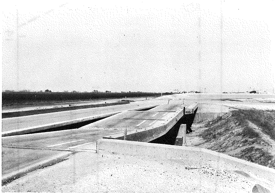
Fig. 57A Photograph of the Bridge 8B After Collapse (through the courtesy of the Transportation Research Board)
