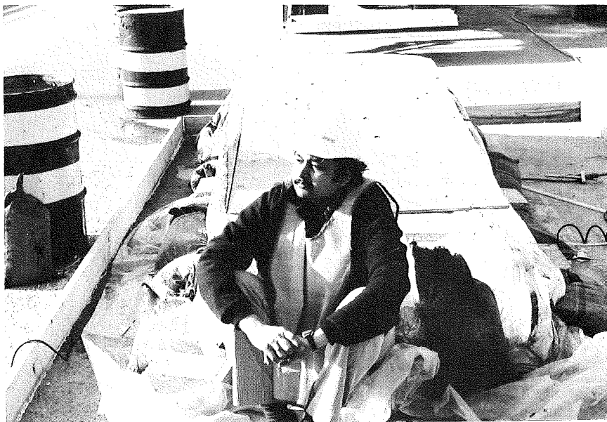
Fig. H-31 Close-Up of Insulated Chamber
