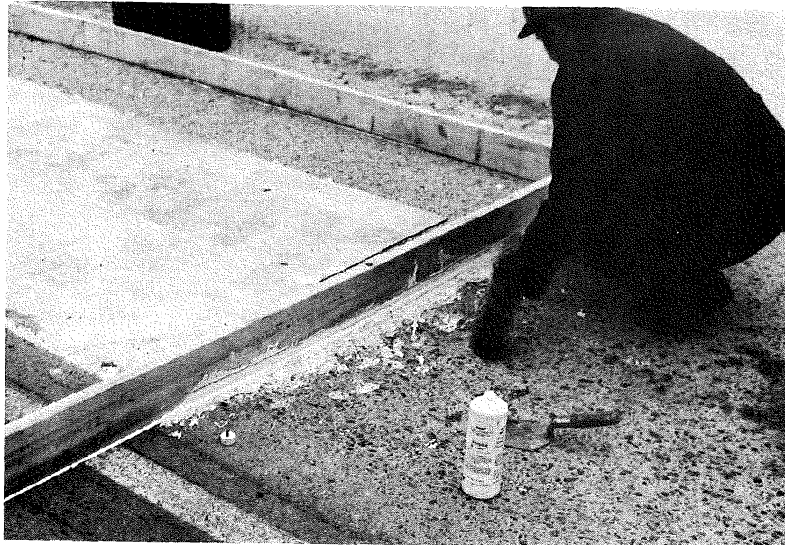
Fig. H-24 Sealing the Dike. Note the Prior Sealing of the Area Already Dried at Left.
