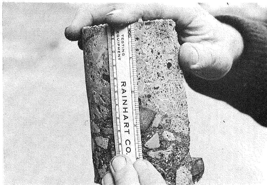
Fig. H-33 Appearance of Acid-Etched Core From Bridge Deck; Note Dense Impregnation to a Depth of 3 Inches (7.6 cm) and Less Dense Impregnation Below
