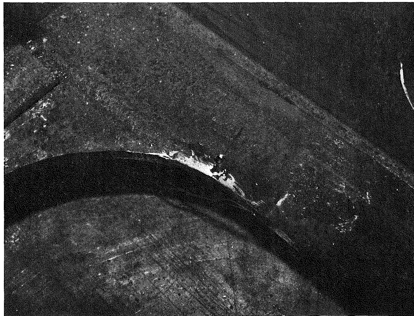
Fig. 58 Typical Fatigue Cracks - Details III ob and IV o
