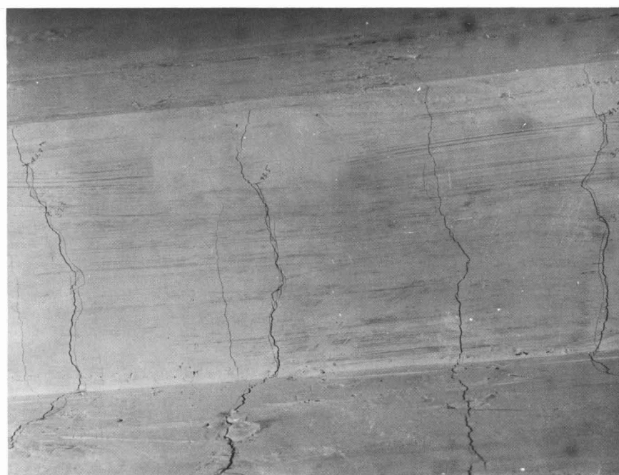
FIG. 49 CRACKING OF CONCRETE, P x -I AT ULTIMATE LOAD
