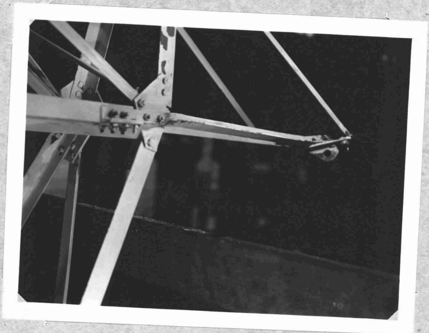
Fig. 6 & 7 - Condition of East Cross Arm at Failure
