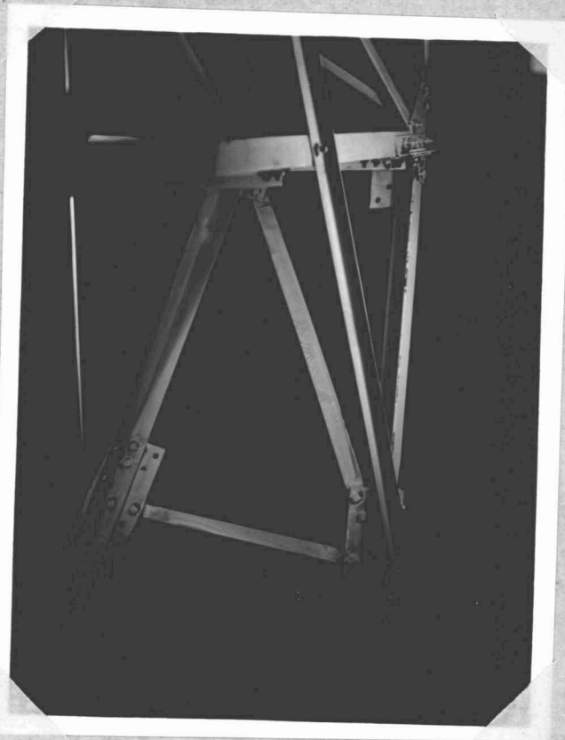
Fig. 8 - Strain Lines in Compression Diagonal (27-39)
