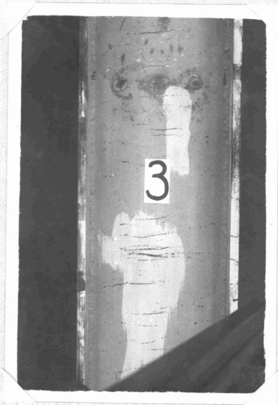
Fig. 33 - Strain Lines on Web of Column 3
