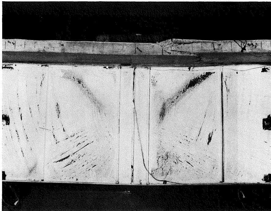
Fig. 10 Failure of Composite Box Girder L1-CB
