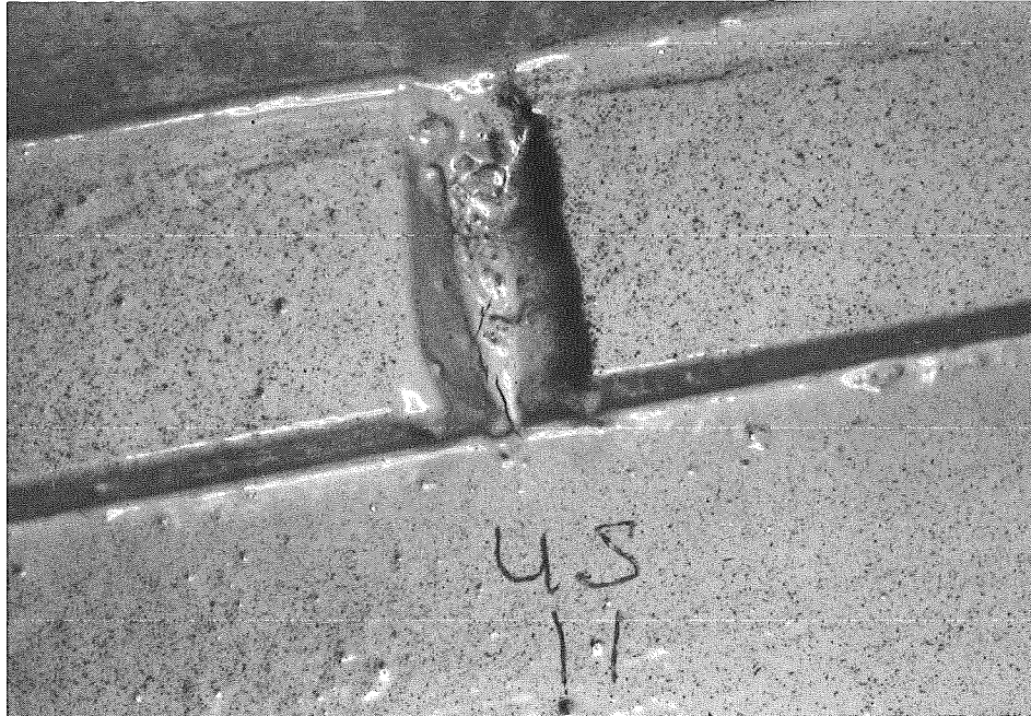
Fig. 74 Crack-like Indication in the Web Plate at Termination of Backing Bar
