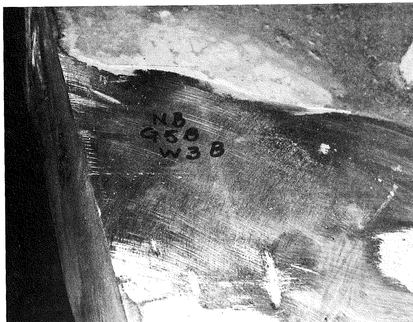
Fig. 3b. Lack of fusion extending across northbound girder G5 W3B about 2 inches.
