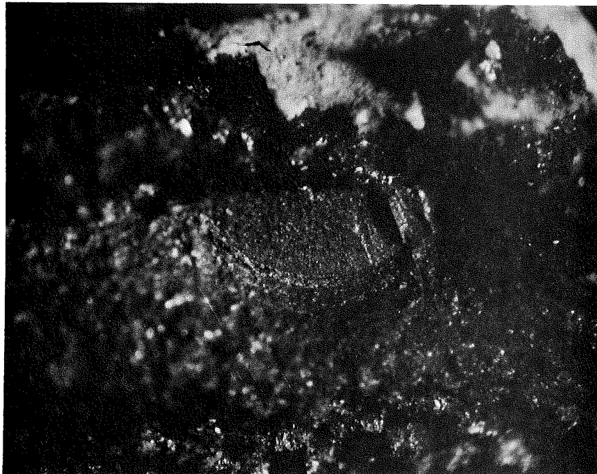
Fig. 21 0.028 inch Deep Crack at the Toe of Type 3 Stiffener-to-Tension Flange Weld (SGC333)
