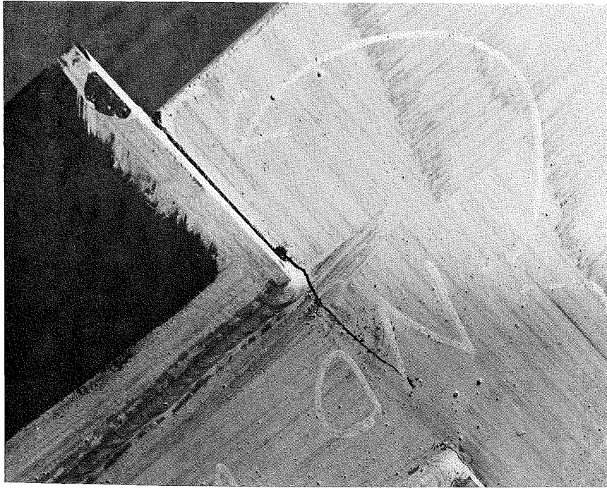
(a) Bottom Flange Surface
