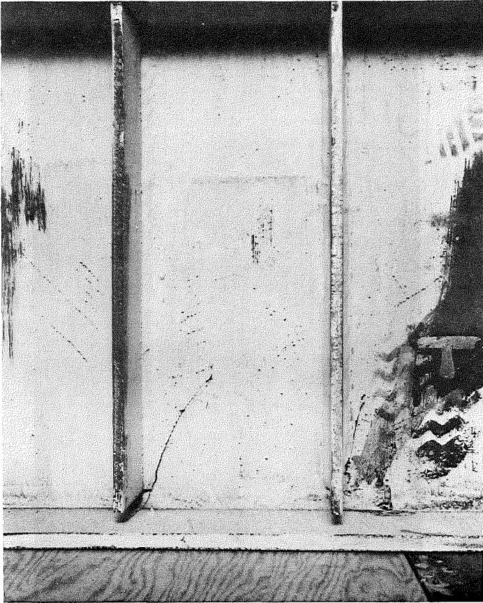
Fig. 12 Typical Failure at Type 1 Stiffener
