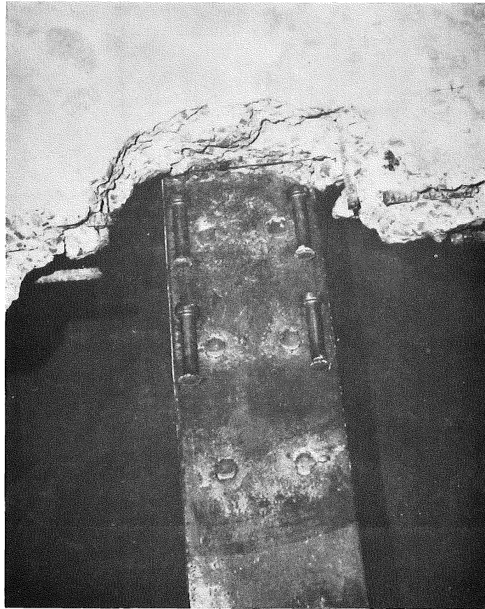
Fig. 15 Studs at the East Inflection Point of Beam CC-1F After Fatigue Testing
