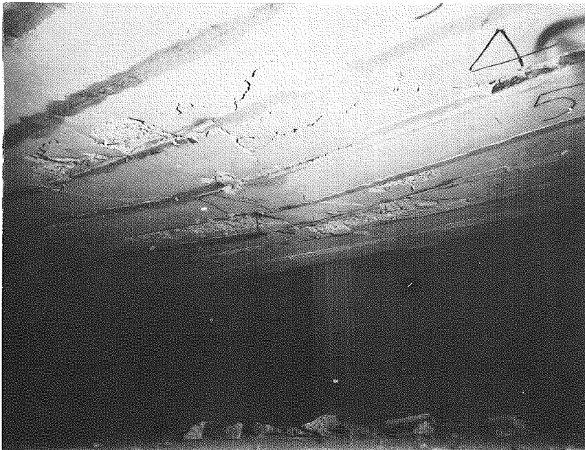
FIG. 24 UNDERSIDE VIEW OF THE BRIDGE AFTER FAILURE
