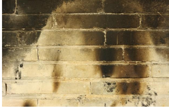
Figure 4.2 An example of soot deposition patterns on the wall after fire is extinguished.
