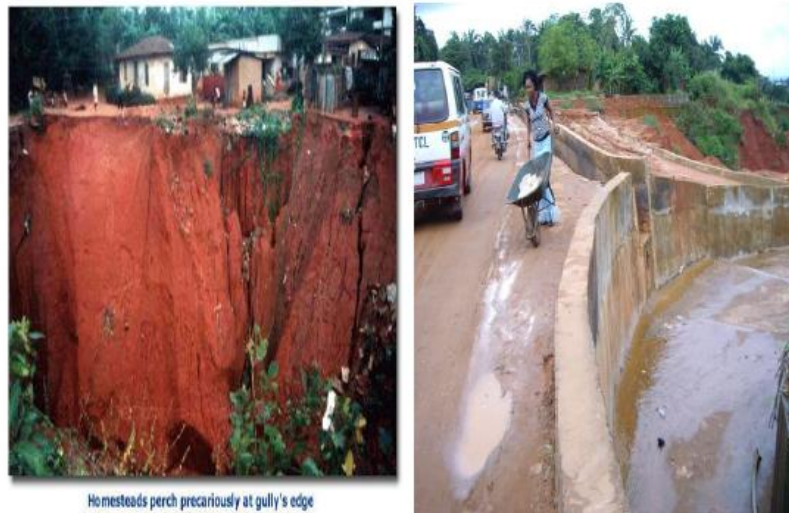
Plate 2 Gully erosion affecting houses and roads in Eastern Nigeria. Source: www.google.co.uk/images (Accessed 05/12/12).
