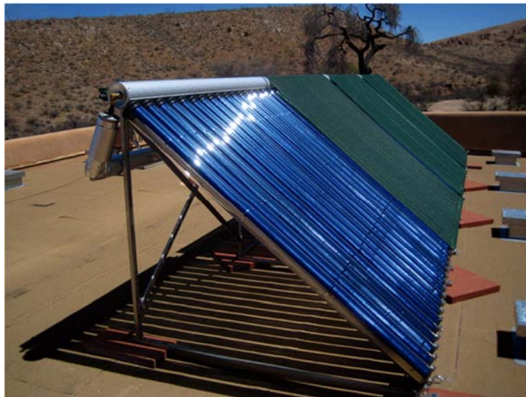
Figure 3.21: Uncovered and covered evacuated tube collectors (Radiant Floor Company n.d.)
