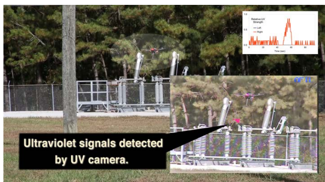
Figure 2. Validation of the compact UV sensor signal with corona camera in a substation measurement flight. The visible camera image shows the UAV above the substation structure (background; UAV is in lightened ellipse). The inset at top right shows the compact UV sensor recording, which reaches a maximum as the UAV passes the corona generator. The inset at bottom right shows the corona camera record; the bright red blobs at the center of the image are locations of UV emission.
