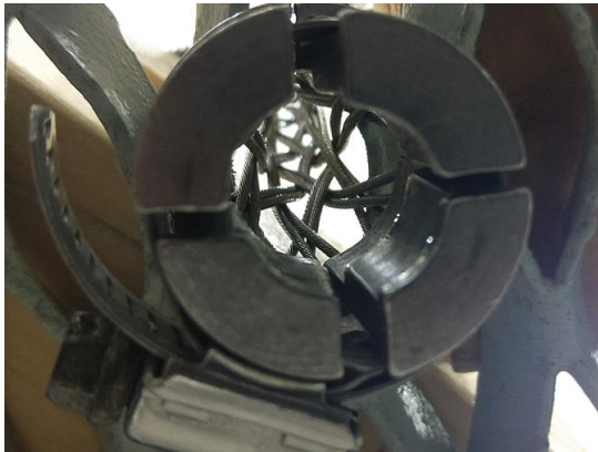
Figure 5. Installed configuration of Kellem. Image credit: Joseph Dziekan, NIFS intern.
