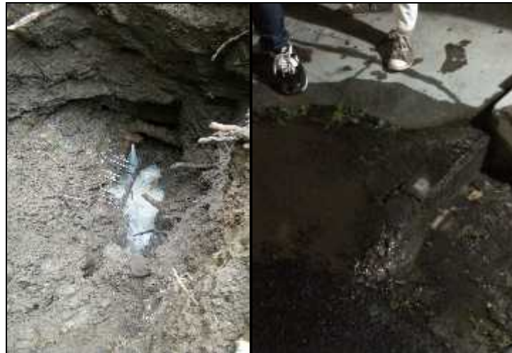
Figure 2. Leakage in Section 4 and Section 7
