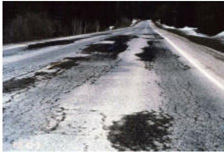
Figure 5. Fatigue Cracking from Frost Action (Washington 2005)
