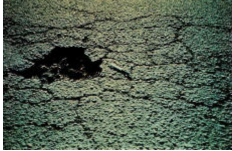
Figure 4. Pothole from Fatigue Cracking (Washington 2005)
