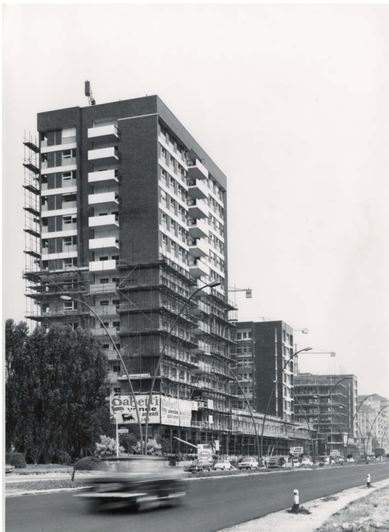
Figure 5. Construction of the 15-storey northern tower in the residential complex of Corso Roma, 1970
