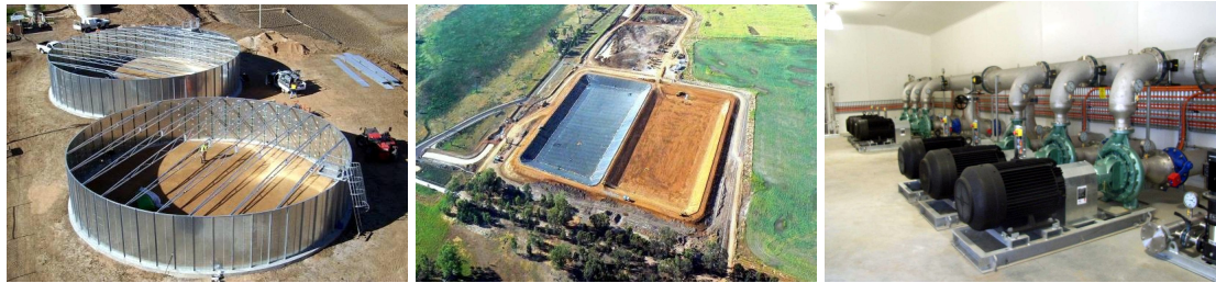
Fig. 4 Wimmera Mallee Pipeline: Left: A typical tank (before lining and roofing). Middle: A typical balancing storage (left lined, right before lining). Right: Pump station.
