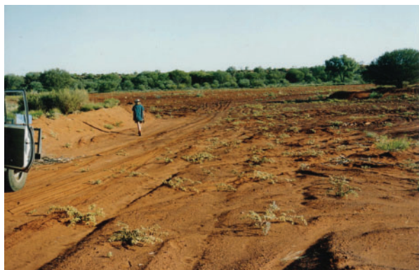
Fig. 3. The sand quarry where the fill for the rehabilitation of the road was sourced. Notice the depth of the soil removed (over 1 metre). Some road areas may have been filled with soil from this depth, hence the poor growth results for some areas.
