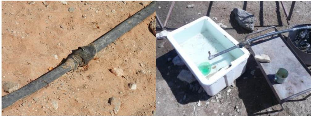
Figure 33: Left: Makeshift Repairs to a Pipe Right: Unclean Collection Containers
