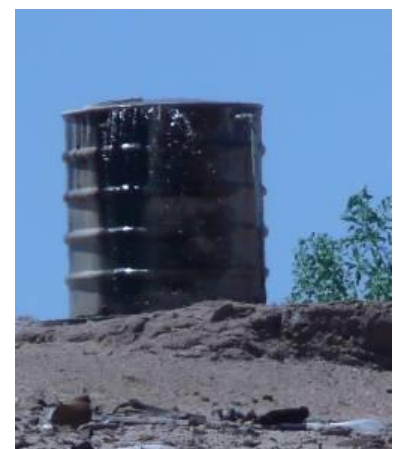
Figure 34: Overflowing water tank
