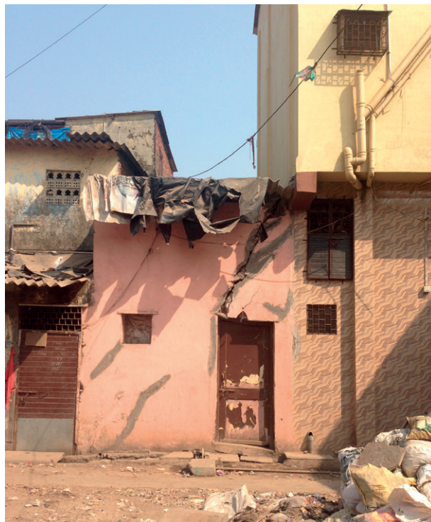
Figure 18 Shifting grounds Newly built and usually heavier houses tend to shift due to the unstable ground in Shivajinagar. Neighbouring houses are affected and walls of older buildings tend to crack under the load. The already fixed cracks re-open as houses continue to sink unevenly into the marshy ground.
