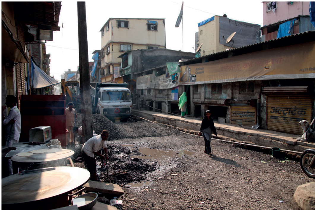
Figure 15 Roadwork (19th December 2015) On-going roadwork raises the terrain. The houses to the right are already half a story below ground.
