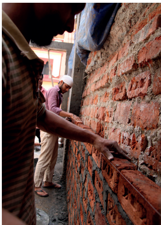
Figure 24 Shared wall - building a double wall At the ground floor a double wall is built up. The bricks are layed on the narrow side in order to save space and money. This indicates double walls are not built for higher structural integrity, but for granting independant buildings.
