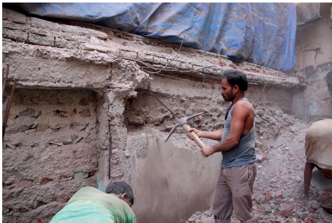
Figure 23 Shared wall - replacing a hard boundary The shared wall between two neighbours is taken down to be replaced.
