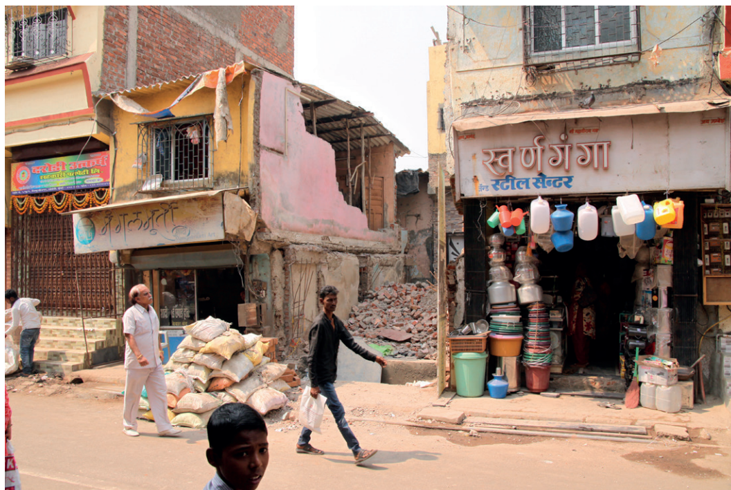
Figure 22 Shared wall The shared wall between two neighbours is taken down to be replaced.
