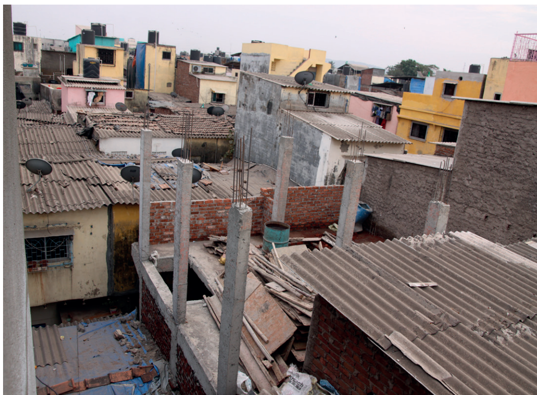
Figure 20 Saving cost by coordinating construction Two plots are constructed simultaneously by two different contractors.
