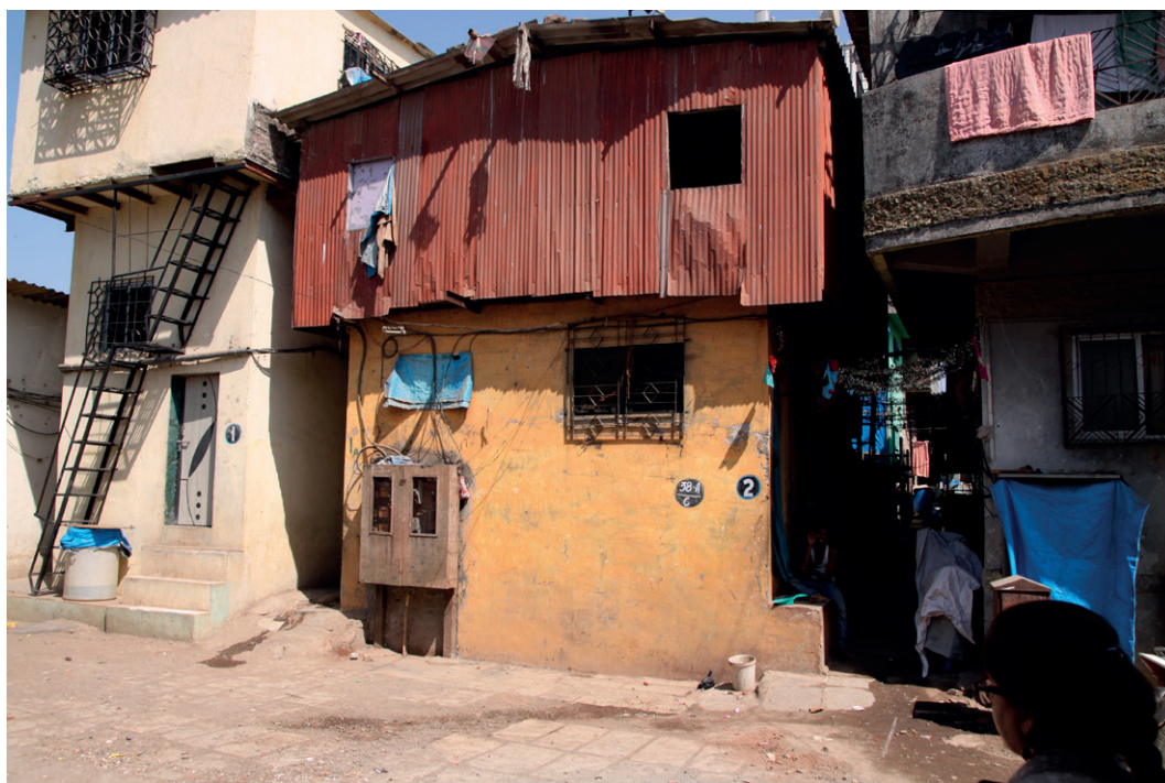
Figure 21 Semi-Pakka construction Rental space on the upper floor with external access, built in katcha material.
