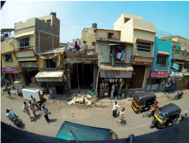
11:50:00 First bricks fall on the street
