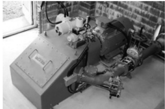
Figure 1 – An Installed Micro Hydroelectric System (Gilbert Gilkes & Gordon, 2014)
