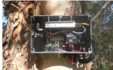
Figure 1: Remote unit with cover removed
