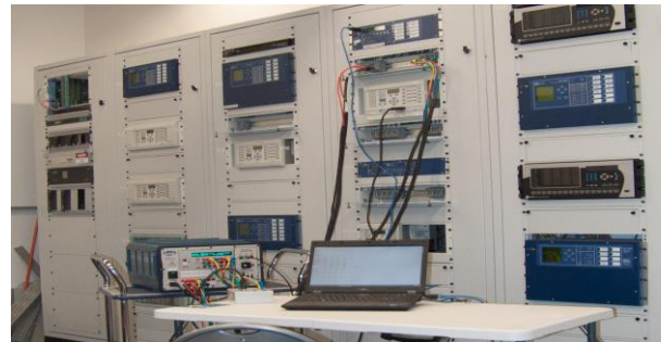
Figure 1 – ActewAGL Distribution SAS Test Facility
