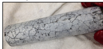
Figure 1: Map cracking in sample
