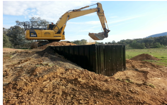
Figure 1 – Excavator and Earth Sheltered Container shipping containers as modular building units and research the general opinion on shipping containers as modular living units and stigmas they may hold. Through data logging and analysis I aim to quantify the impact earth sheltering and other passive heating and cooling methods have on the thermal performance of a shipping container.
