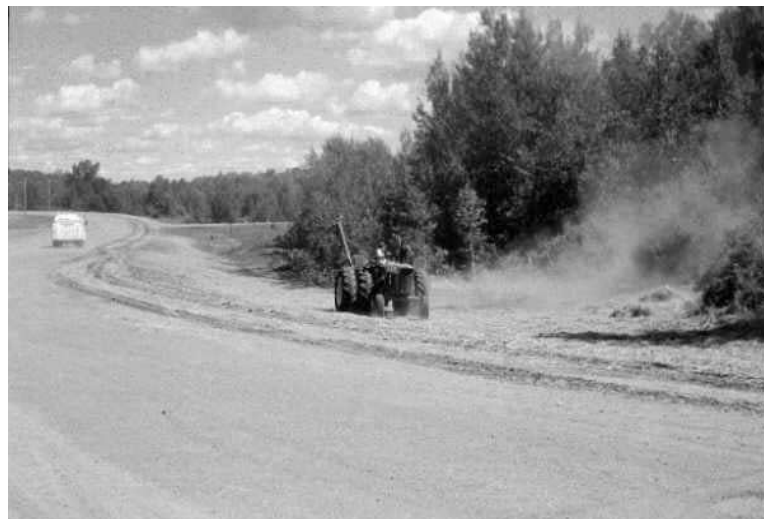
Mulch protects seed and soil from erosion until vegetation can be established.
