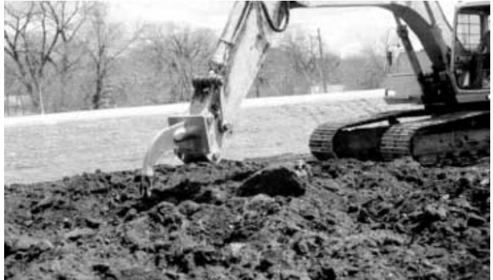
Scarifying the soil during construction significantly improves the chances of any vegetation establishment.
