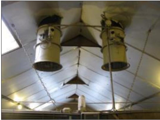
Ventilation fans (room with traditional floor)
