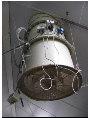
Ventilation fan (room with manure belt)
