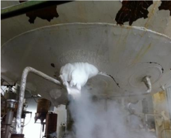
Fig. 1. Photo of the B-1 tank with cracks
