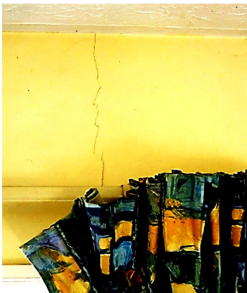
Figure 10: Vertical crack above window corner existing prior to testing, Wairoa St. Photo D. Yeoh
