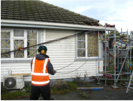
Figure 5: Applying load to the house via the chain block, Bexley Rd. Photo H. Morris
