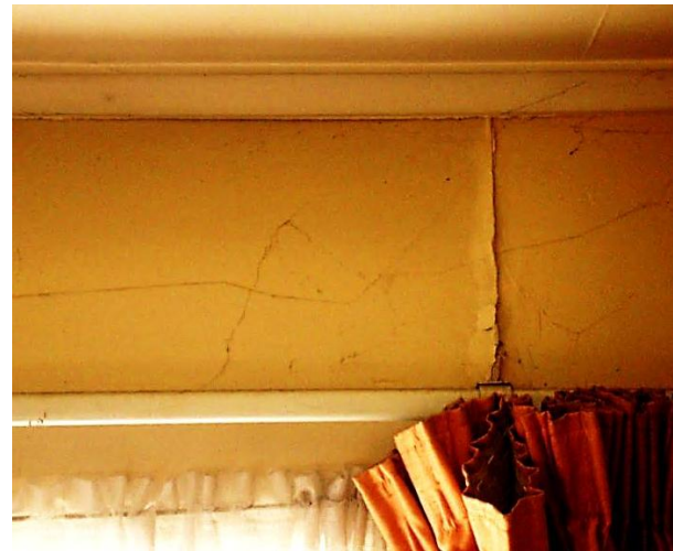
Figure 21: Buckling of wall lining above window at 130kN load, Bexley Rd. Photo: L. Holt
