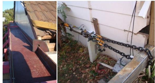
Figure 8 The 360 UB 57 Load beam positioned at ceiling against the gable end(a left). Load cell and reaction chain looped around RHS at floor level (b right). Wairoa St.
