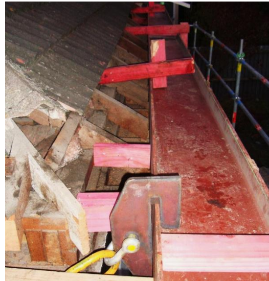
Figure 2: Load beam with slide plate with 90x45mm props to transfer load to the top plate, Bexley Rd. Note a string line along the outside edge used to monitor beam bending. Photo: L. Holt
