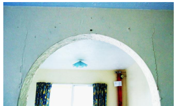
Figure 17: Arched opening in central bracing line of Wairoa St while under 100kN test load. This existing damage was enhanced by the application of the test load.
