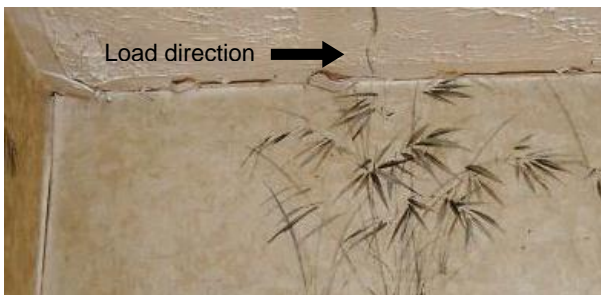
Figure 19: Cracking showing movement between ceiling and wall at 130kN load, Bexley Rd. Photo: L. Holt
