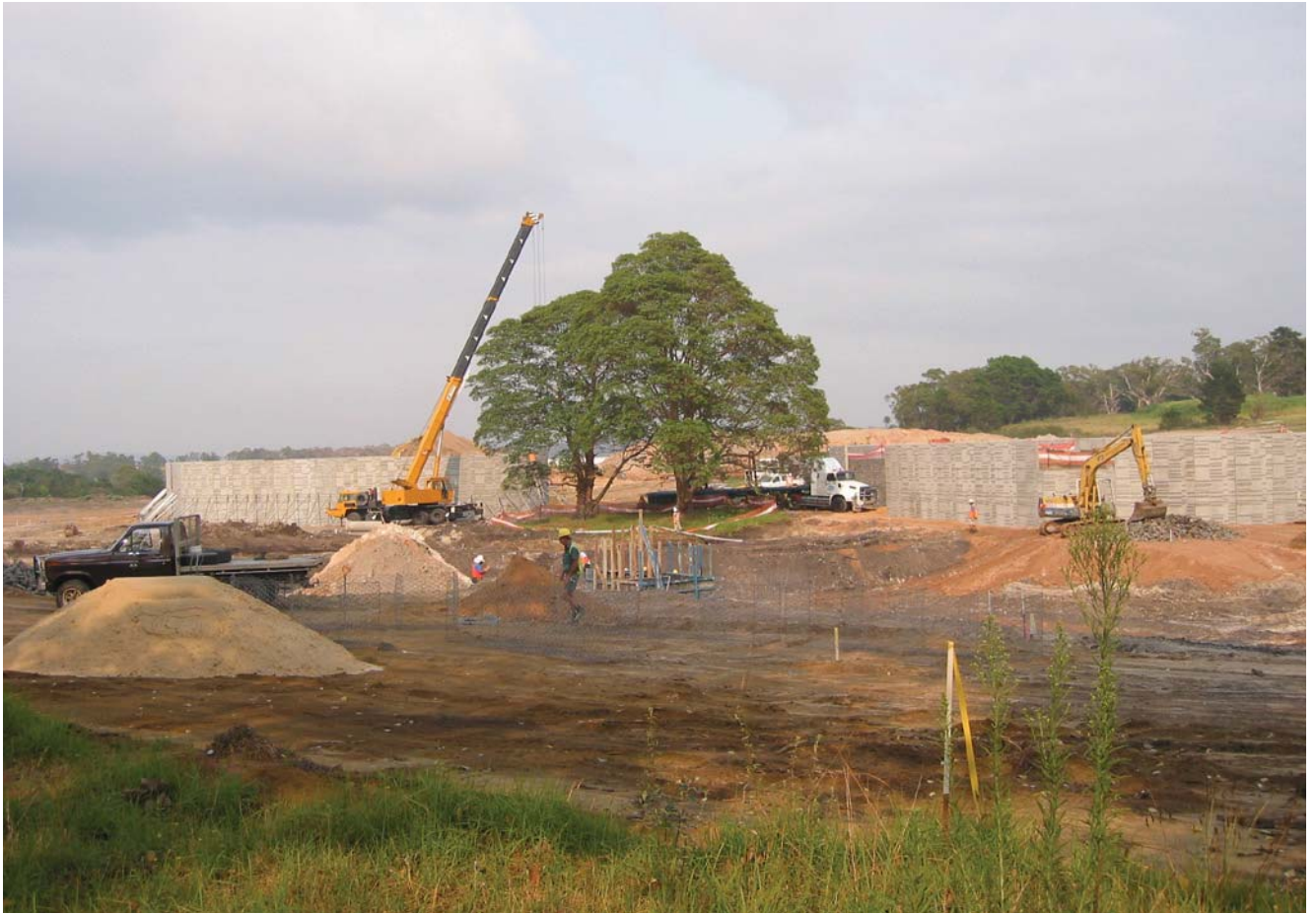
Construction photos. The Plateau asserting itself as a figure in the landscape
