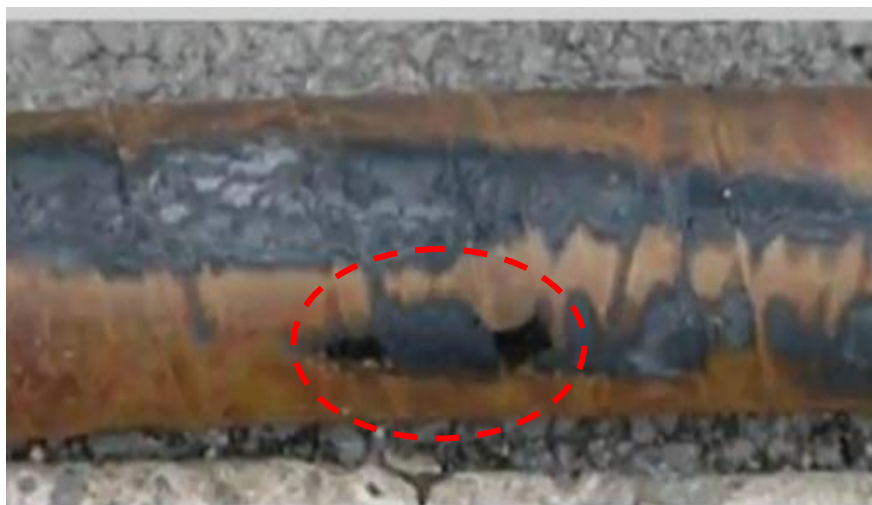
Figure 2.5: Defect of power cable because of Ageing
