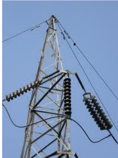
Figure 1.1 : Insulators in high voltage transmission line
