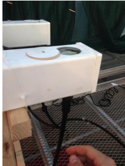
FIGURE 21: OVERFLOW FROM CLOGGING
