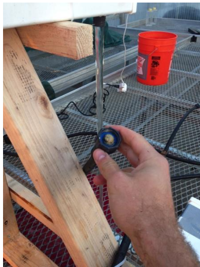
FIGURE 22: CLOGGED MESH FILTER
