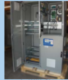
2 x 125Vdc-75A with battery cabinet
