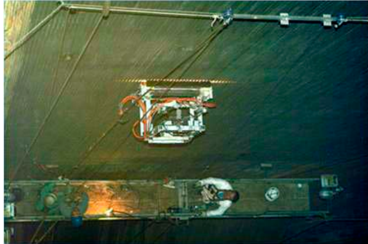
Figure 13.2-6: Inspectors on a scaffold watch the LaRC patented thermal line scanner they implemented for boiling water power plant NDE.
