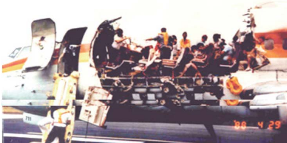
Figure 4.3-1: Forward fuselage after Aloha Airlines accident (1 person killed), April 28, 1988. Fuselage of Aloha Airlines Flight 243 after explosive decompression.
