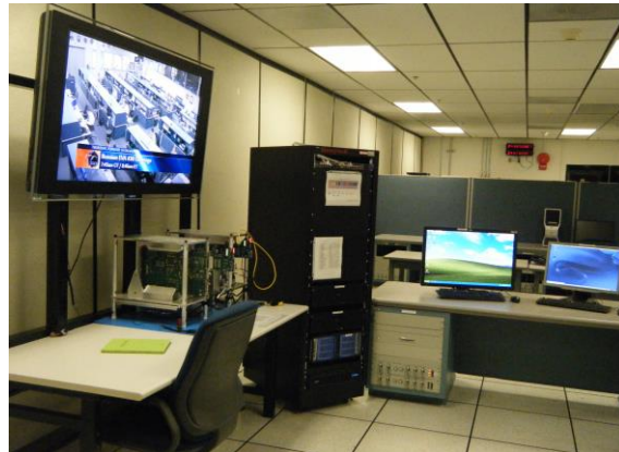
Figure 1 - CAIDA Lab in SSPF with Honeywell Test Bench and Orion VMC
